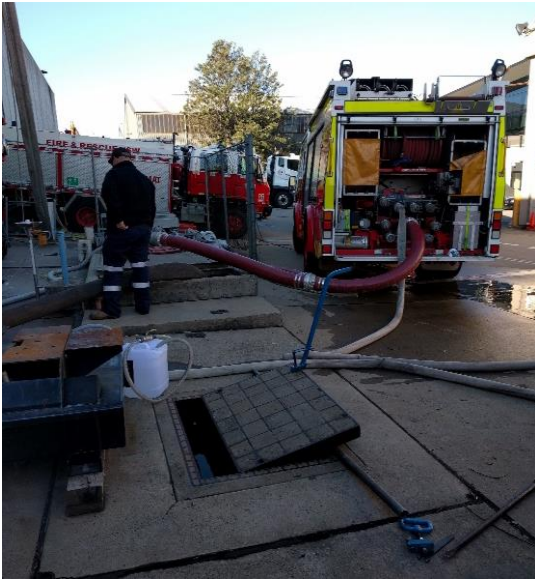
Photograph 1: Second retention tank pit identified (FW02), showing a truck connected to the above ground recycled fire water tank (FW01)
