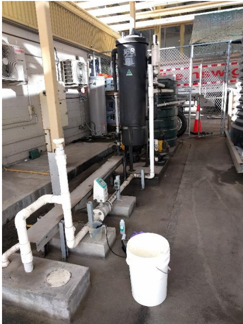
Photograph 12: Site interceptor system (sampled as SW08), showing water holding tanks in the background, leading to the discharge point in the foreground.
