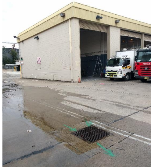
Photograph 2: Sample location SW05 facing towards MW02, showing the incoming and outgoing drainage channel directions from SW06 and a down pipe on the truck wash, to SW04.
