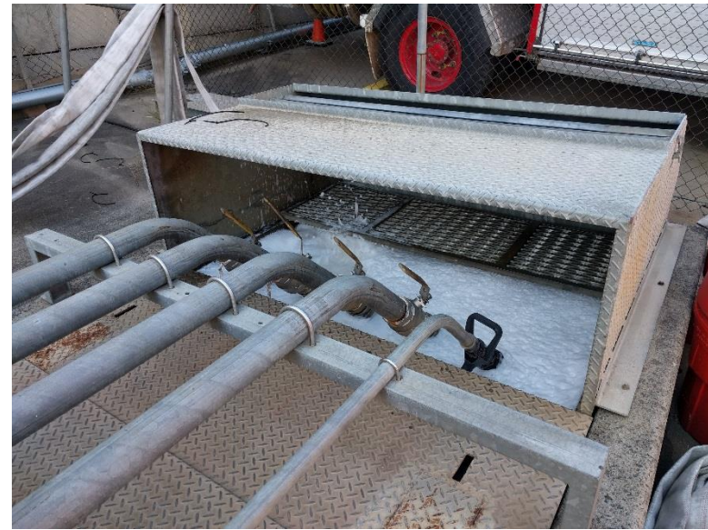
Photograph 4: Fire retention pit foaming after accidental discharge of foaming agent from a truck into the pit.
